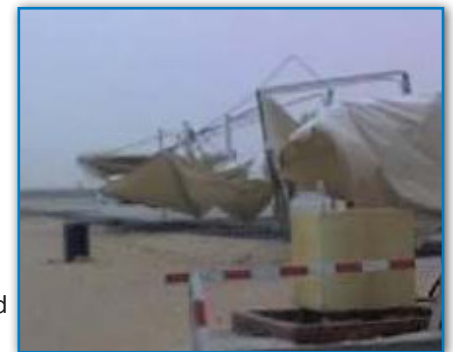
Wind Damaged Car Shade
